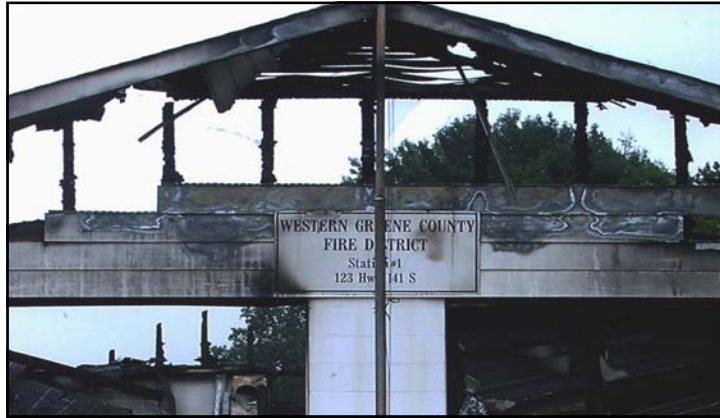
The Western Greene County Fire Department received $15,000 to rebuild their fire station community building after it was destroyed in a fire.
